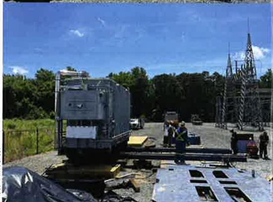
The transformers on their way to Wye Mills.
